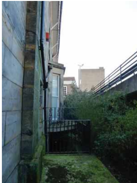
View along the rear elevation of no. 10 showing the bay window and the proximity of the multi-storey car park.
