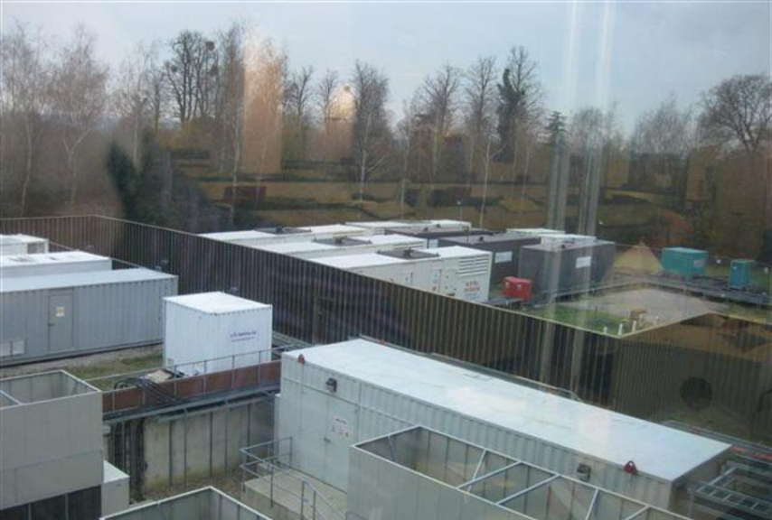
View of plant from inside data centre
