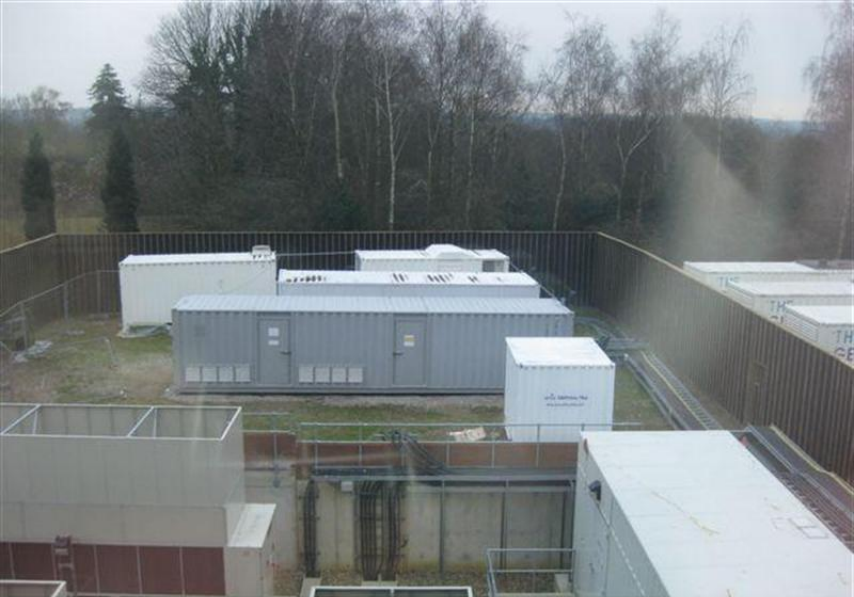
View of plant from inside data centre
