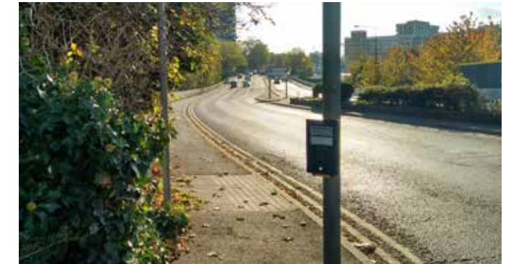
3.4 View south along east side of Wat Tyler Way showing existing shared use footway
