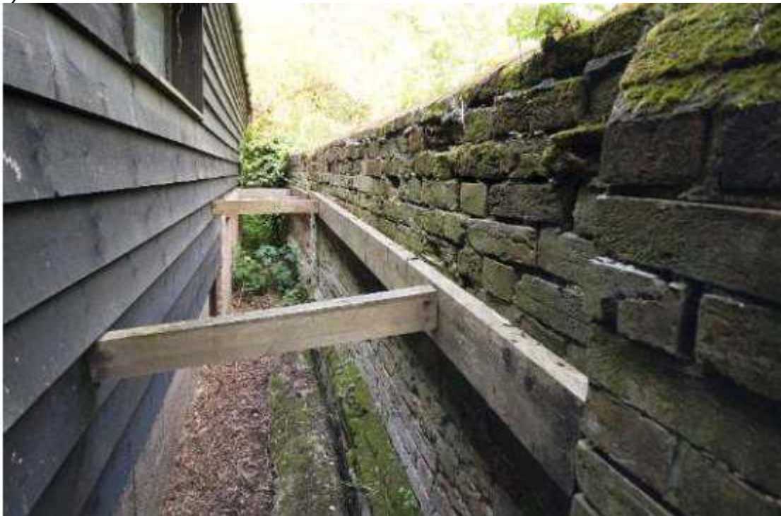
Figure 10 South wall curtilage listed showing existing propping (prior to its partial removal)
