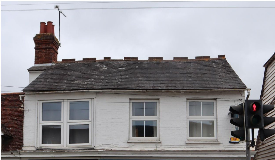
Figure 46 - UPVc double glazed windows change the character of the building, and cause harm to the Conservation Area.
