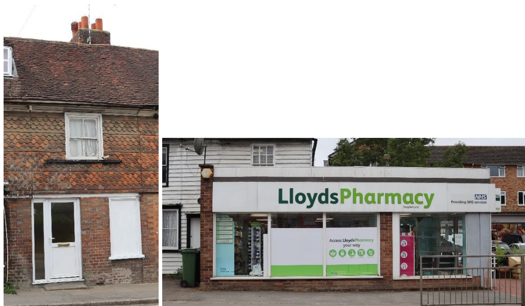
Figure 48 – UPVc door (now replaced and blanked window to a traditional building and poor shop front which forms part of a listed building.
