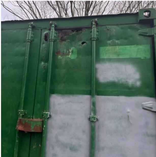
Image 1: Visible corrosion on the existing unit.
