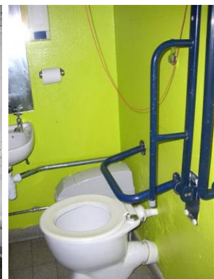
Brenchley (Alarm cord)
