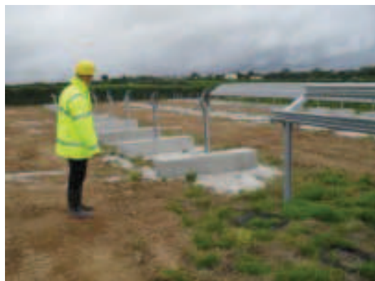
Where there are areas of archaeological interest, and therefore a need to avoid ground disturbance, the use of precast concrete anchors should be considered, as shown here at the 5MW Trefullock solar farm in Cornwall.
