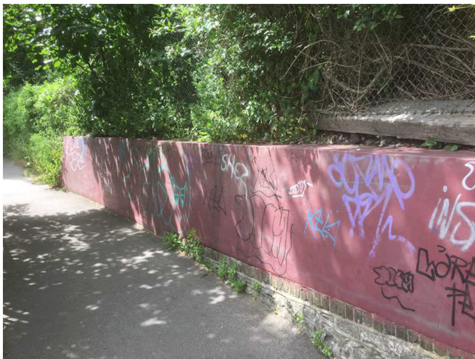
Photo 2: Graffiti along High-Level Bridge
