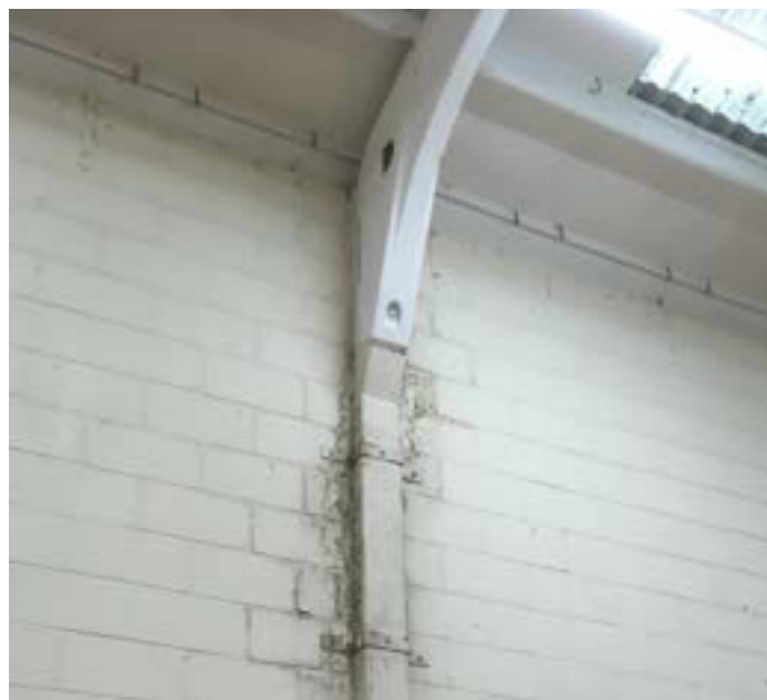
Image F- Evidence of leaking internal rainwater pipes
