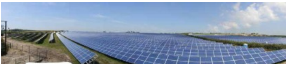
Solar PV facility adjacent to Saarbruecken airport.
