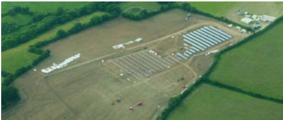
Construction of the 1.4MW solar PV farm on land adjacent to the Hendra Holiday Park, Newquay. Images courtesy of the Hendra Holiday Park.
