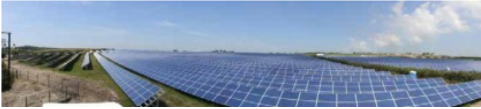
Solar PV facility adjacent to Saarbruecken airport.
